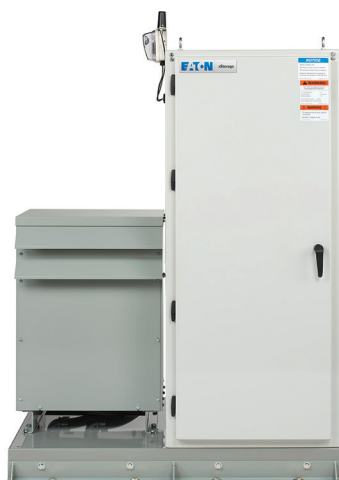
Control cabinet with 480/208V auxiliary transformer
