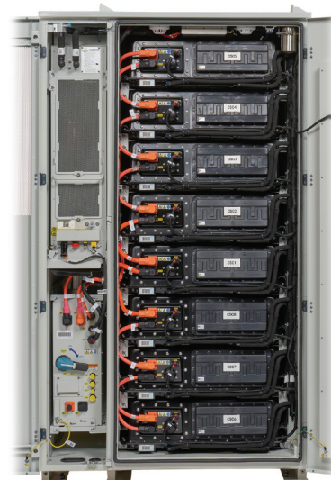
Battery cabinet (interior view with 8 battery modules)
