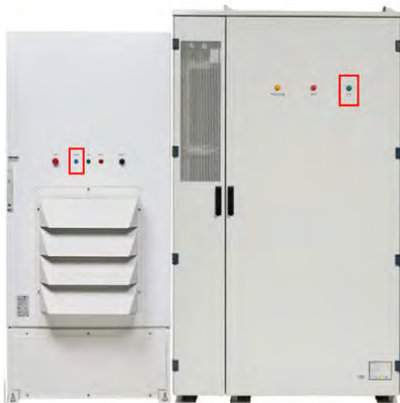
Figure 68. Inverter and Battery Auxiliary Power Indicator Locations
