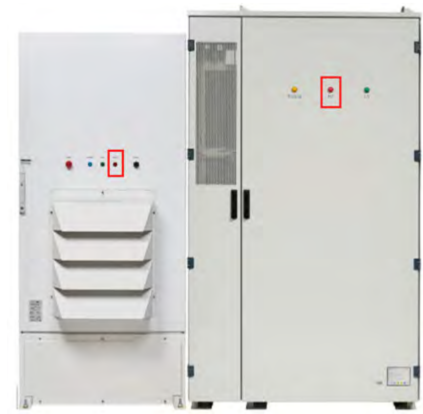
Figure 70. Inverter and Battery Run Indicator Locations
