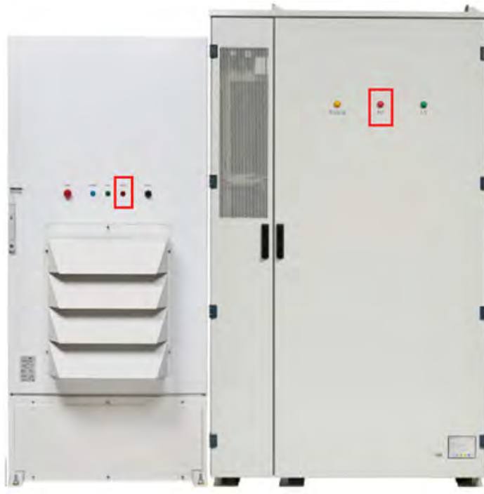
Figure 75. Inverter and Battery Run Indicator Locations
